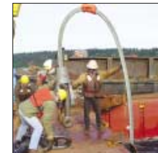
A short section of 4" chain connects the 3.5" bridge strand to the anchors.
