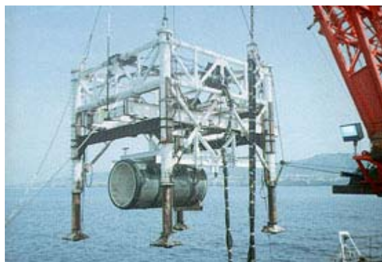
First replacement concrete pipe section during lowering with "horse" at Point Loma.
