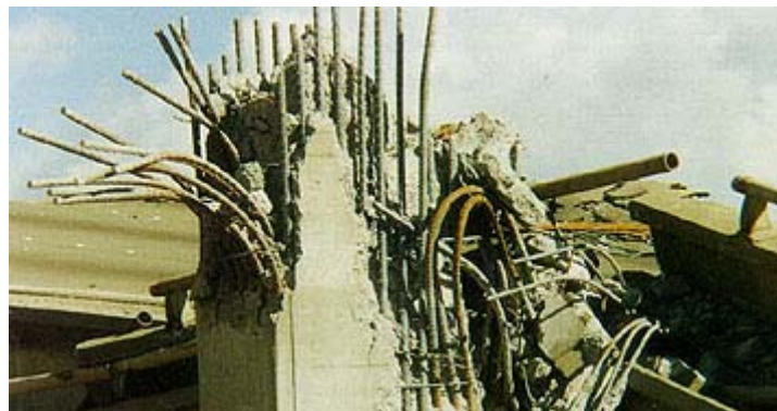
Shear failure of Cypress Double Deck Freeway
