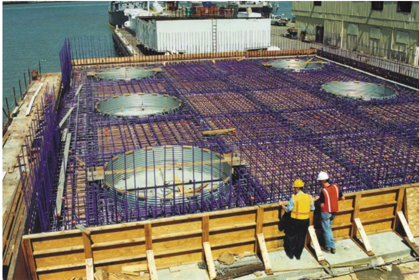
Casting of float-in cofferdam for Installation of drilled shafts for support of the four main tower legs of the New Carquinez Bridge, Crocket, CA.
