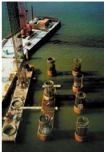
Installation of drilled shafts for the new Cooper River Bridge, Charleston, SC.
