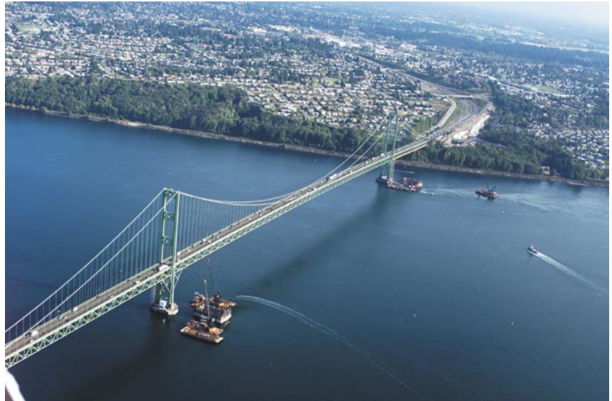
Aerial view of the two caissons moored alongside the existing bridge comprising the foundations for the new bridge.
