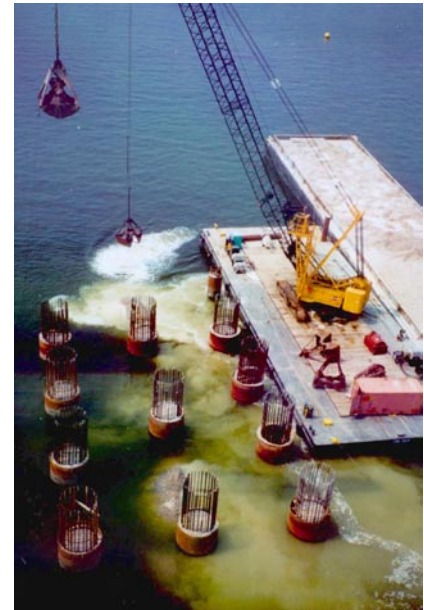
Placement of rock for pier protection islands on the Cooper River, Charleston SC.
