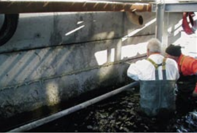
The Faro Bridges - cathodic protection as preventive maintenance strategy for the bridge piers.
