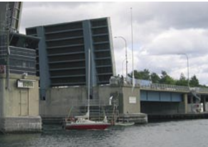
Egersund Bridge - cathodic protection as repair strategy for the bridge piers above and below water.
