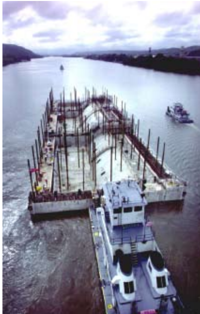
Float-in of Segment 1 from casting basin to outfitting pier. Braddock Dam, Pennsylvania
